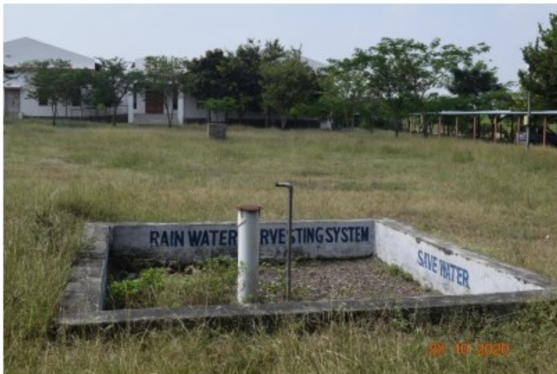
Rainwater harvesting System to Recharge Bore well at college campus
